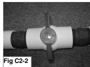
Valve in the closed position Solar heating is ON ( heating )
